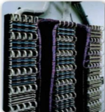
Infrastructure de local technique
